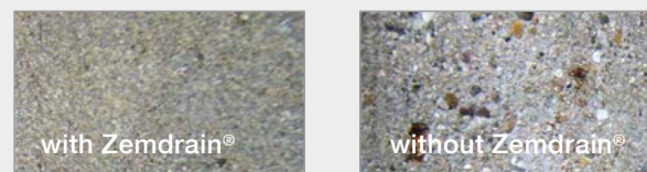
Picture 1: Visual difference between concrete walls produced with Zemdrain® and without Zemdrain® at the walls of the wastewater treatment plant Offenburg after 10 years of operation.
