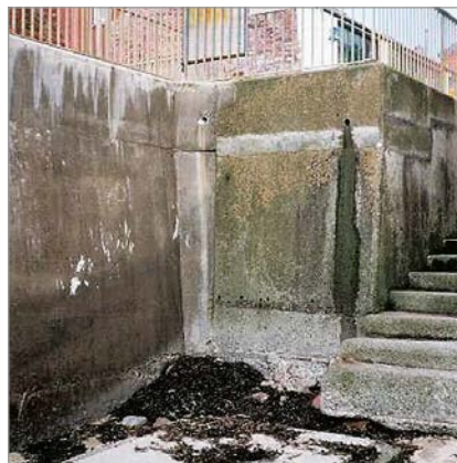
Concrete surface degraded by abrasion and microbiological growth)
