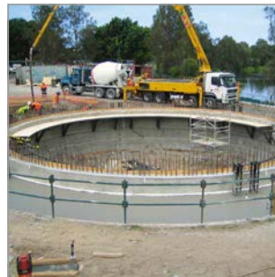
Pumping Station, Gold Coast (AUS), 2007
