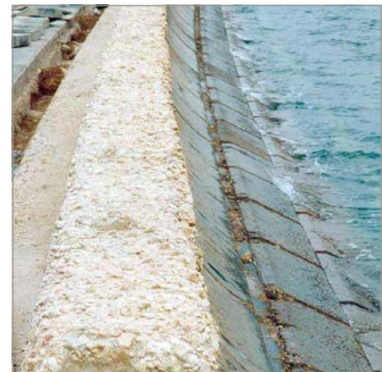
Concrete surface degraded by sea water
