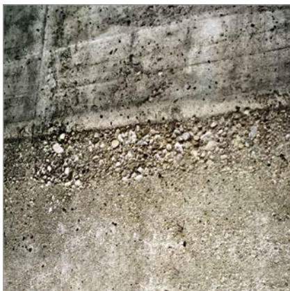
Concrete surface degraded by wastewater
