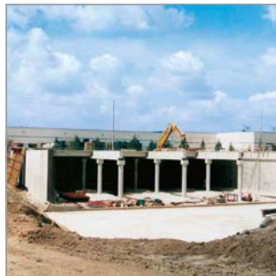
North Meadowvale Reservoir and Pump Station, Ontario (CA), 2006
