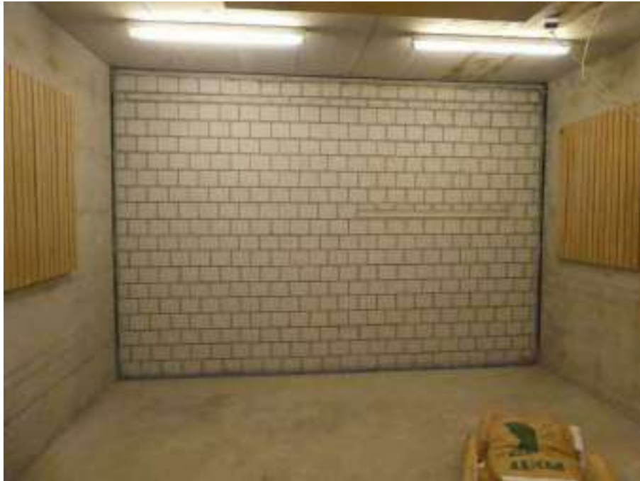
Figure 26: View of the wall as seen from the source room. The stair landing and the stair flight were not yet installed.
