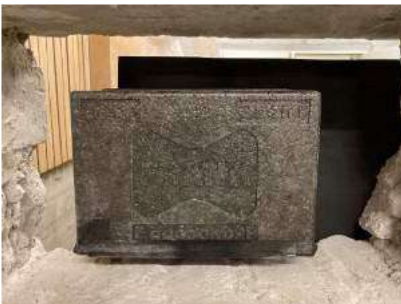
Figure 19: Installation situation of Egcosono SP stair landing bearing with 15 mm elastomer bearing
