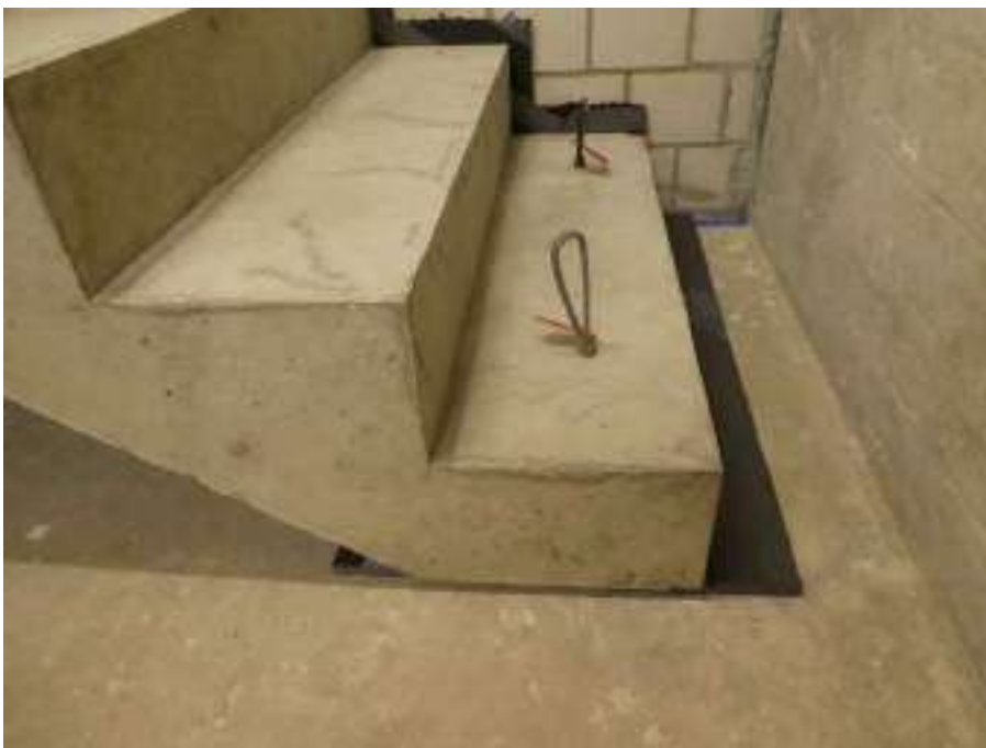
Figure 17: Staircase bearing Egcoscal SP F-shape for load level 43 kN in installed state (below)
